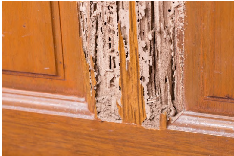
Household timber ravaged by termites
